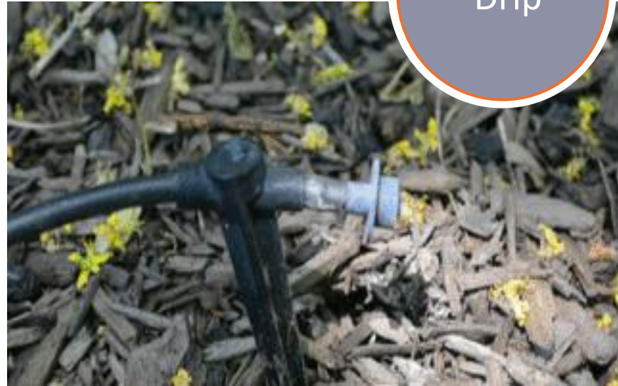
Point Source Drip
